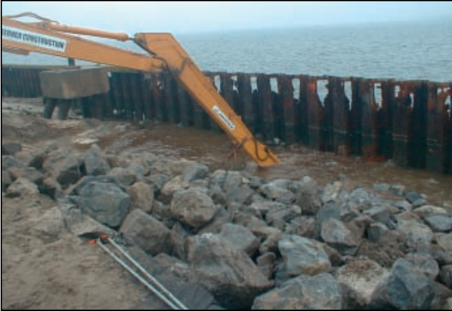
The first task was removal of the steel sheet seawall, which had badly deteriorated. Photo credit: Berner Construction, Inc.
