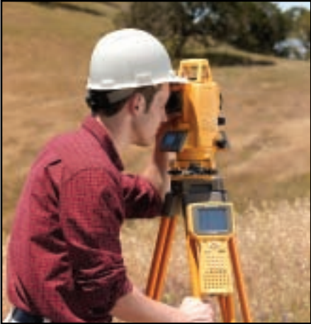
A Topcon GTS-236W Electronic Total Station and RL-H3C Rotating Laser were used to hold and check grade during the process of placing rock in 25-foot sections. Photo credit: Topcon Positioning Systems.
