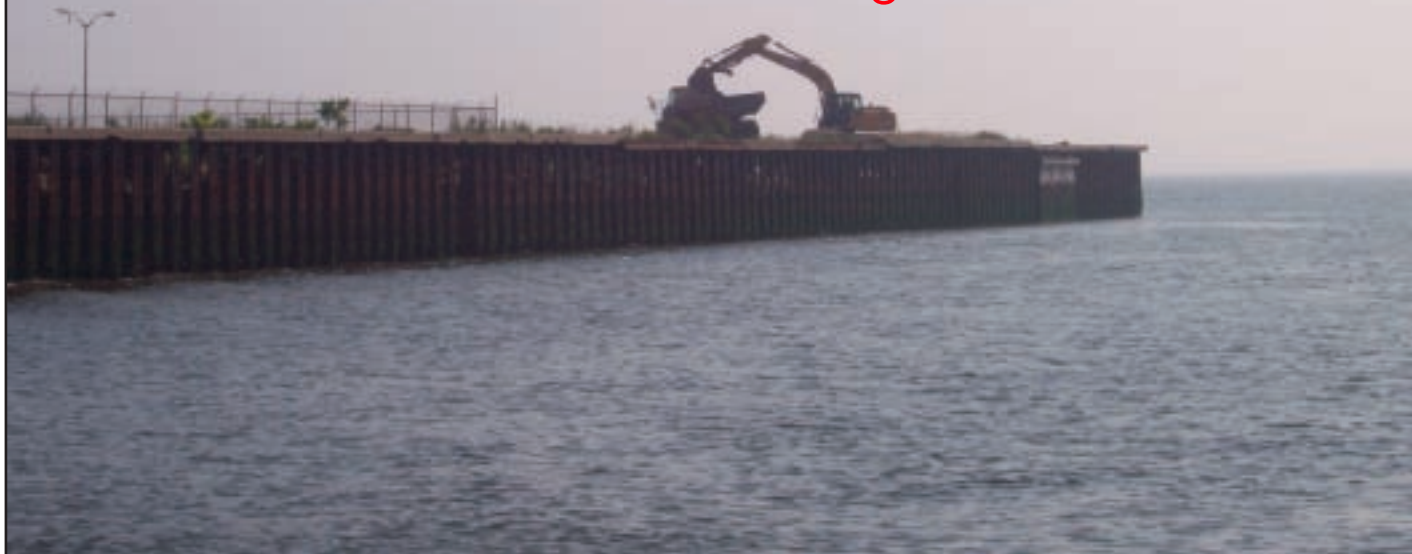
The shoreline at the Floyd Bennett Field Marine Corps Reserve Center in Brooklyn, N.Y., recently required stabilization after experiencing considerable erosion that damaged a parking lot and posed a safety hazard. Photo credit: Berner Construction, Inc.
