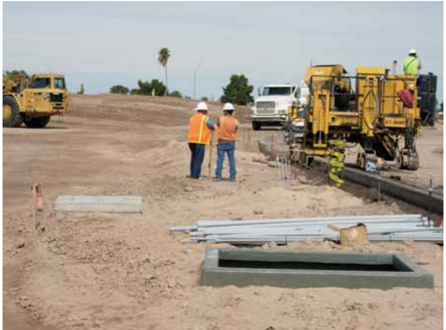
Haydon Building Corp. installed pipe for potable water, sewer force main, gravity sewer and storm drain at a field maintenance shop in Florence, AZ.
