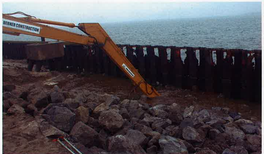
The first task was removal of the steel sheet seawall, which had badly deteriorated.
